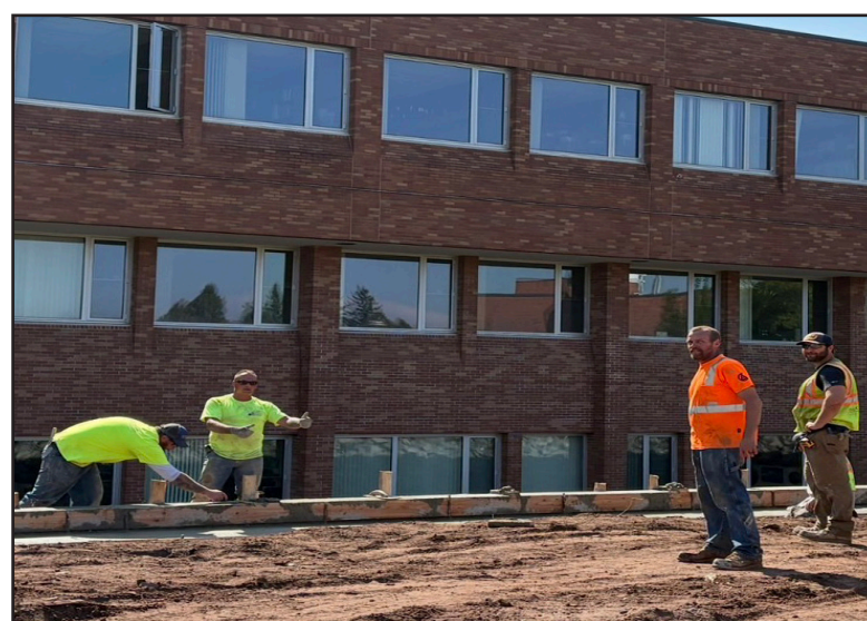
Construction workers building a fence in front of Holden Fine Arts on Sept. 15, 2025.
