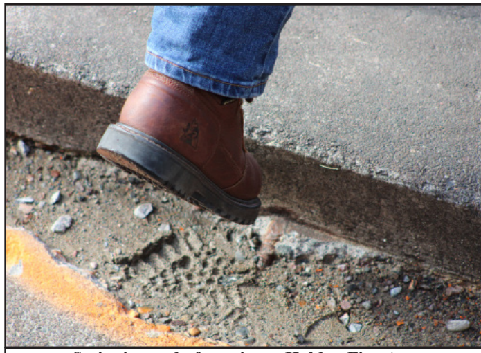
Stairs in need of repairs at Holden Fine Arts
